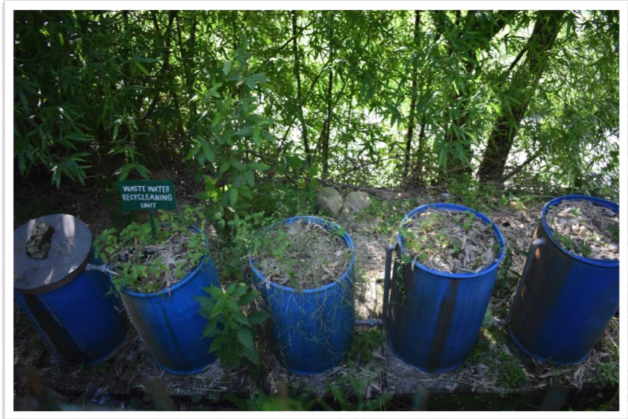
Image of a Waste water recycling and cleaning unit
